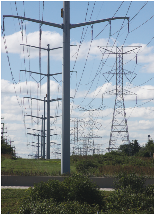
Figure 6: Non-contact measurement captures infrastructure without shutdown. A recent application for a natural gas distribution company required analysis of electrical transmission lines that traversed the gas company's assets.
